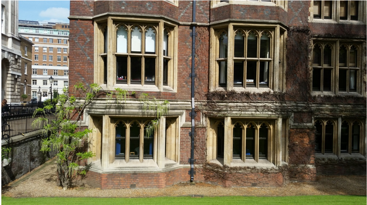
Existing Western elevation (NW corner of building) – Showing existing wisteria (supported by wire system). And Ivy which has started to die back.
