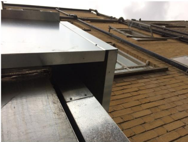
View of stainless acoustic screen around fan motor at rear, looking up towards top of flue above roof.
