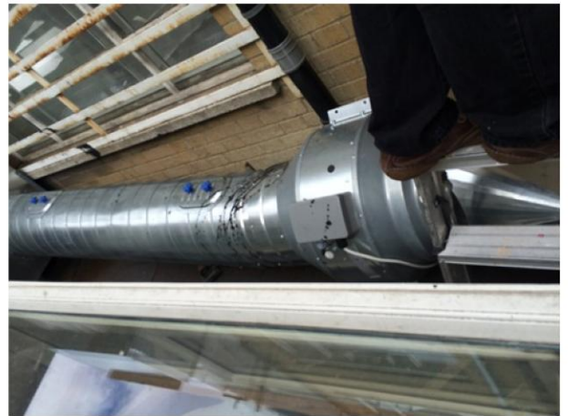
View of new fan motor, and horizontal duct, unscreened, near skylight.
