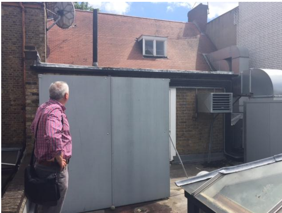
Photo 4: AC units hidden behind acoustic screens
