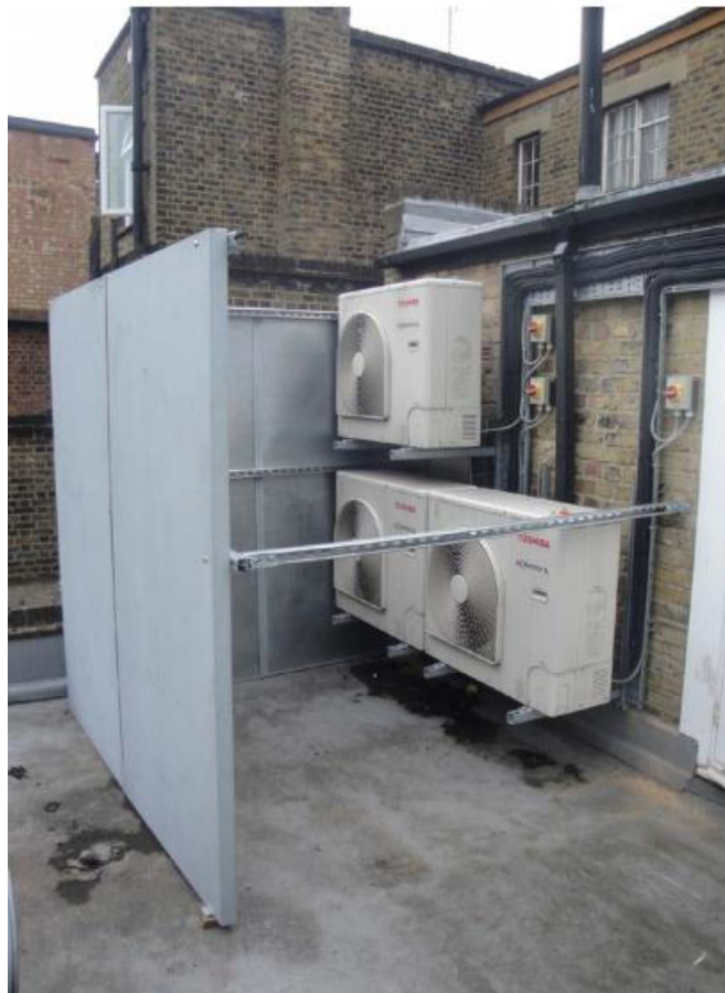
Photo 6: Existing equipment and acoustic screens
