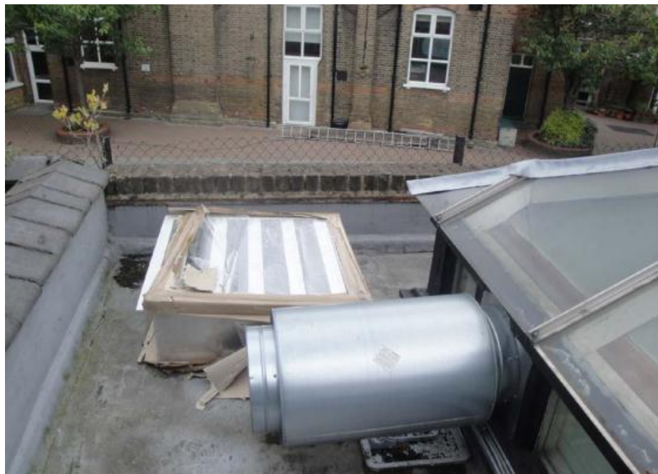
Photo 8: Rear parapet of the application property partly shields the equipment
