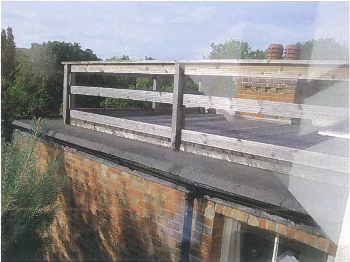
Existing unsafe third floor roof terrace
