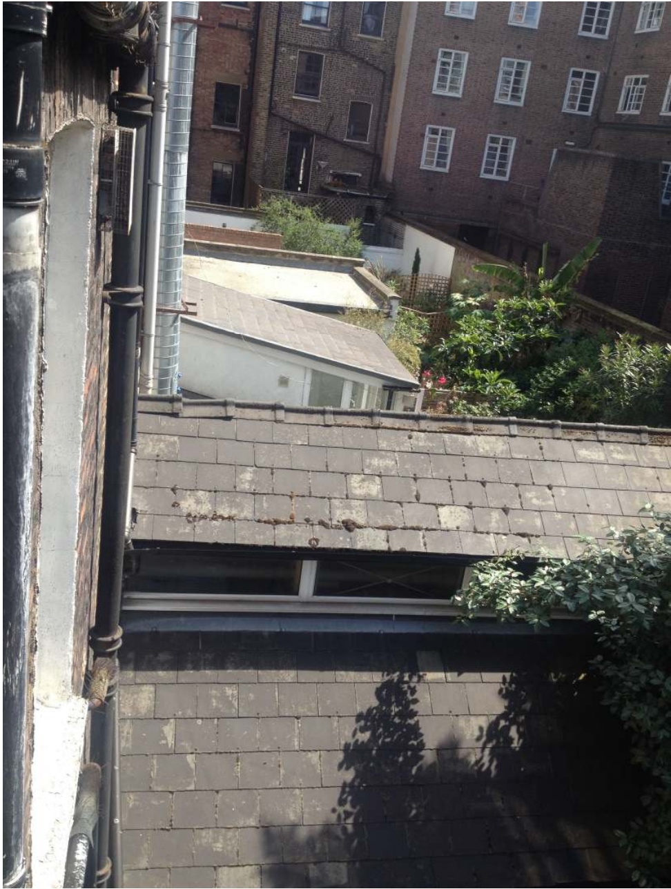
PHOTO 9: The numerous rear extensions and alterations along the terrace to the east
