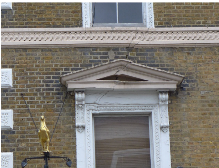
Structural repair required to first floor front head.
