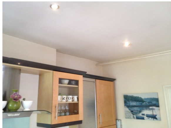
[10] Second Floor kitchen showing no cornice
