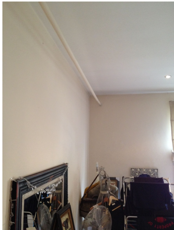
[13] Second Floor rear bedroom showing no cornice
