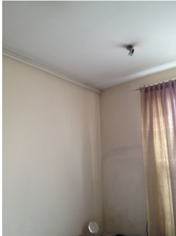
[7] First Floor rear bedroom no cornice
