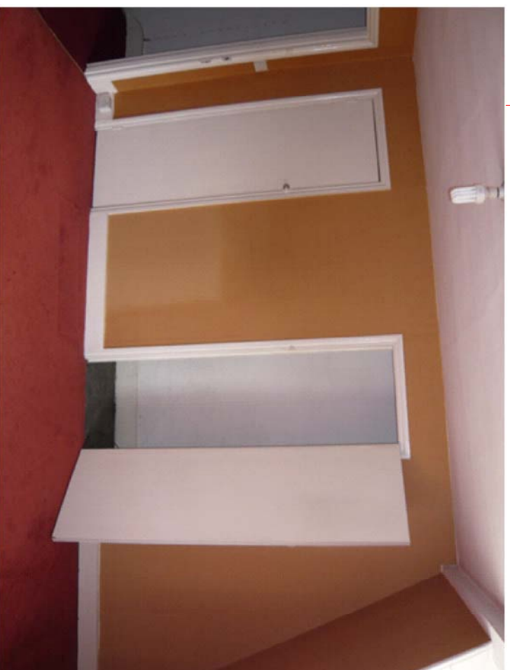
Remove new stud wall and doors and reinstate to large open room.
