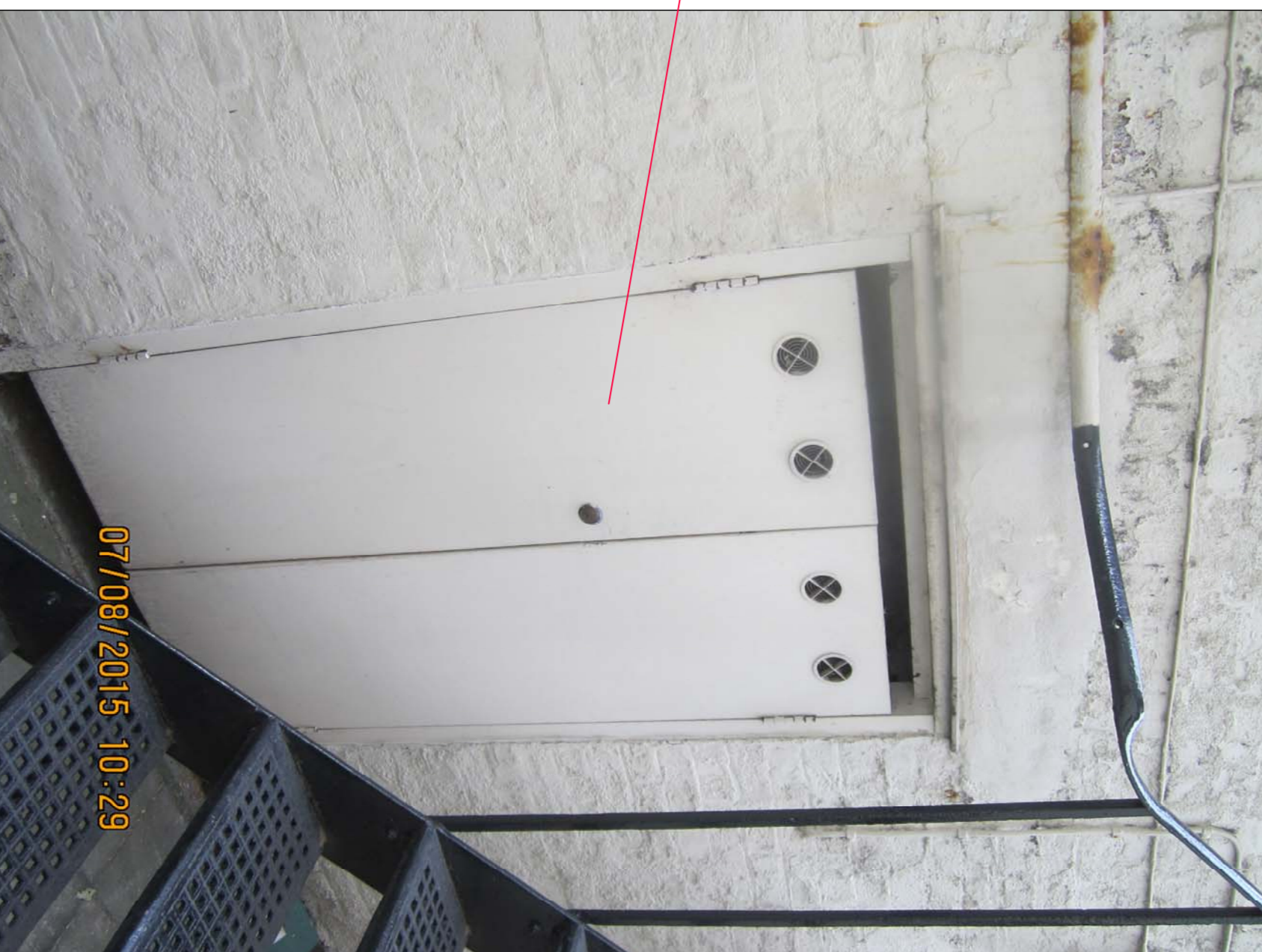
DOOR 3 EXISTING RIGHT SIDED DOUBLE DOORS LEADING TO VAULTED AREA BELOW GOWER STREET (N15)
