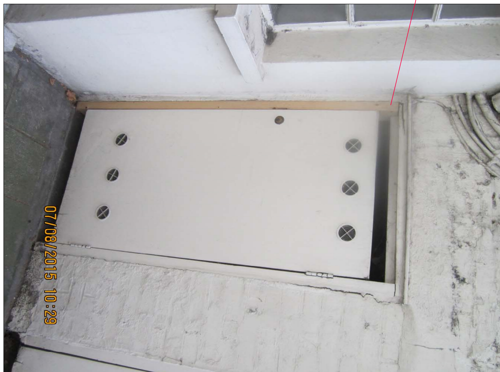
DOOR 1 EXISTING LEFT SIDE DOOR LEADING TO VAULTED AREA BELOW GOWER STREET (N15)
