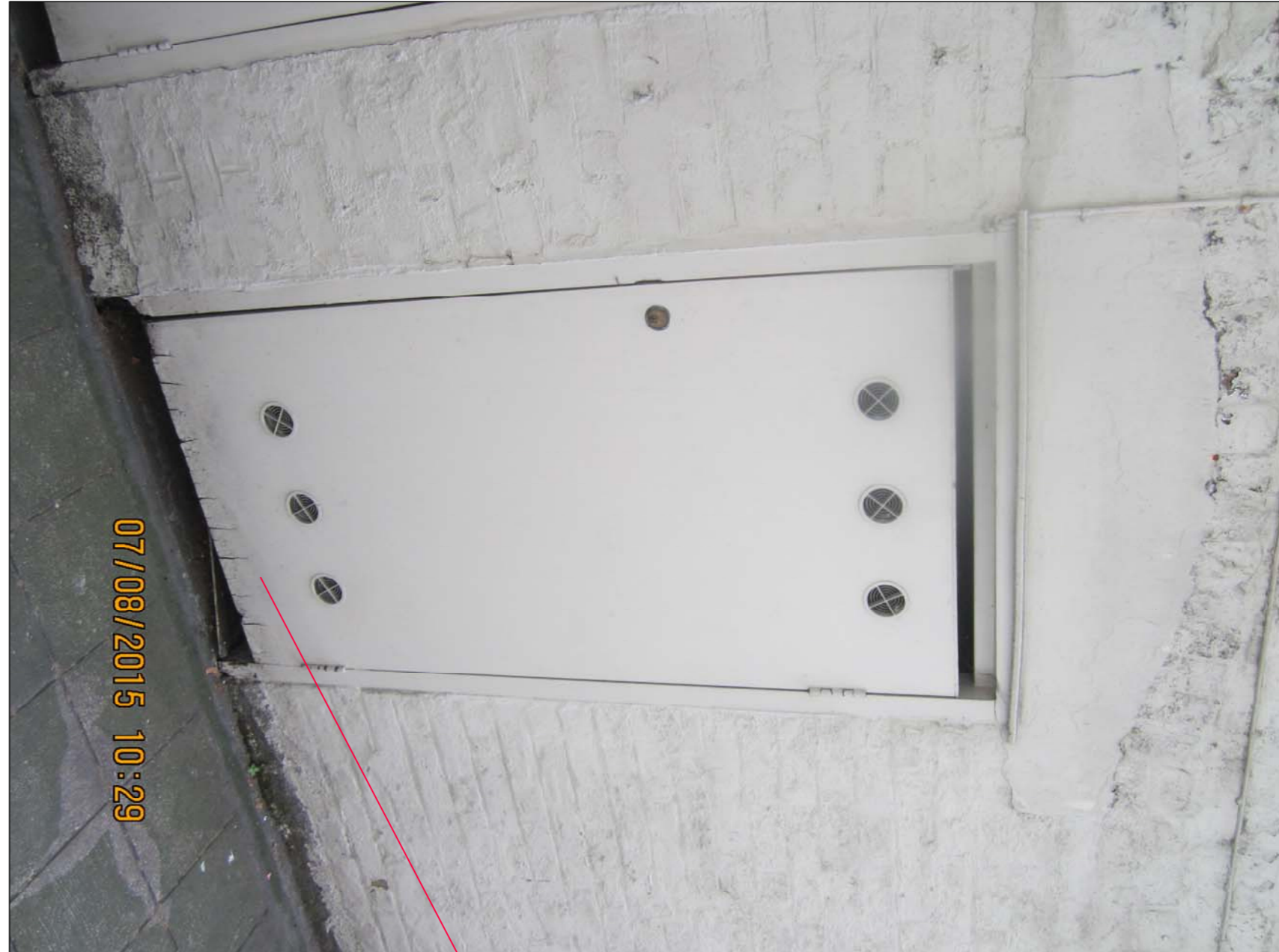
DOOR 2 EXISTING MIDDLE DOOR LEADING TO VAULTED AREA BELOW GOWER STREET (N15)
