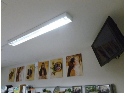
SURFACE MOUNTED FITTING SOUTH SIDE OFFICE AREA.
