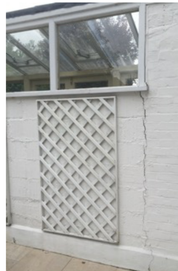
03. party wall is of poor construction and showing signs of cracking
