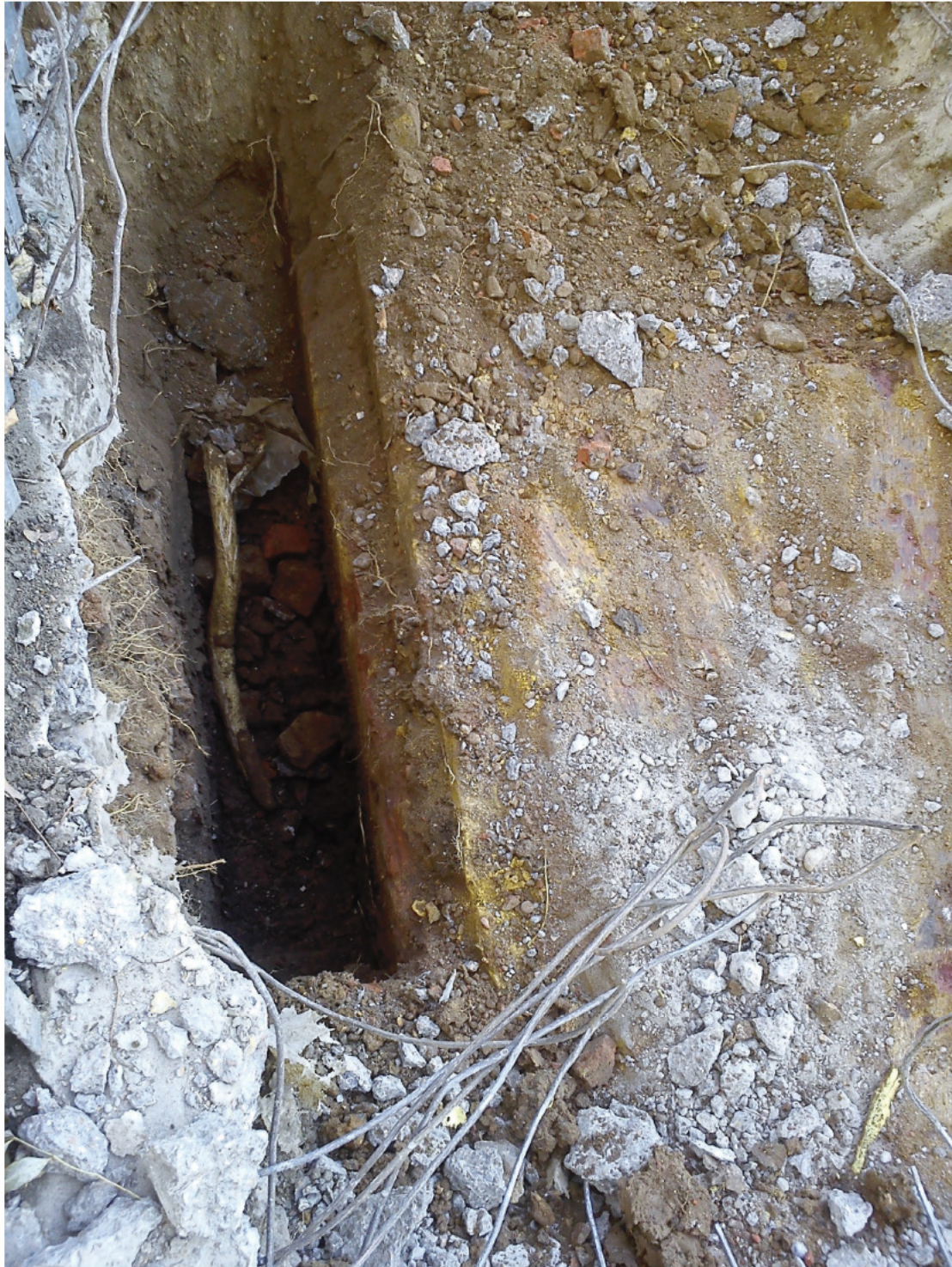
Photo 1 – TP301: Brick Wall Encountered
