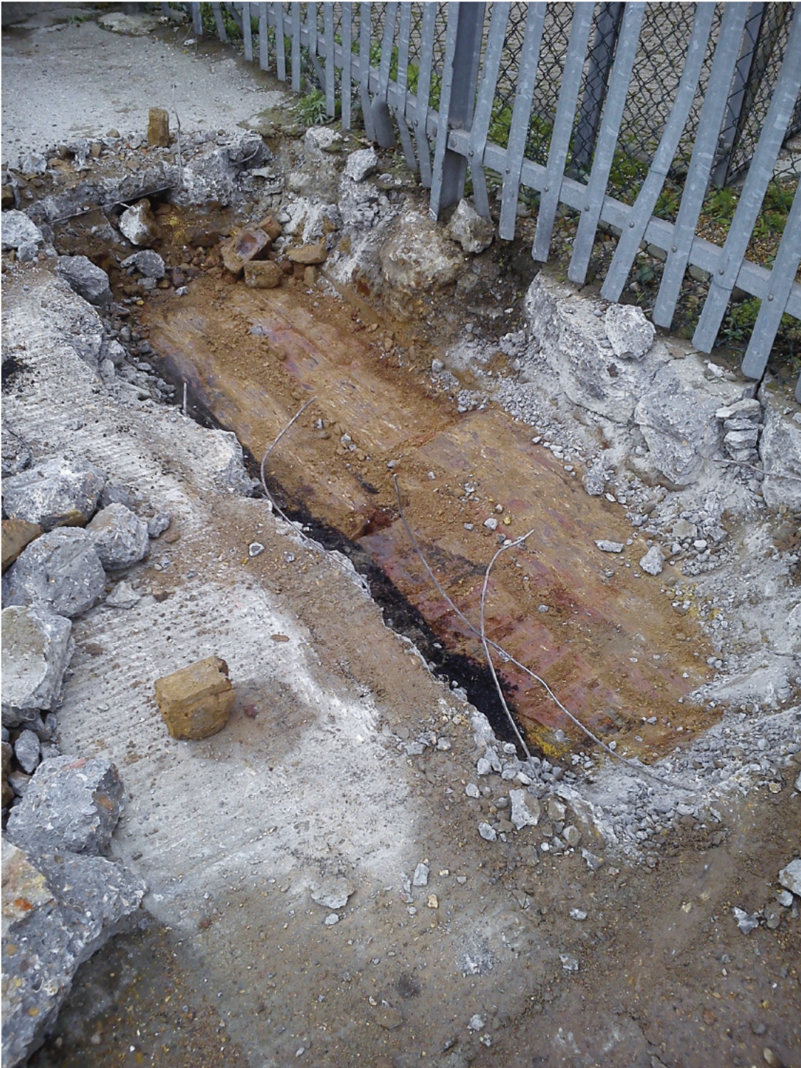
Photo 3 – TP303: Brick Wall Encountered
