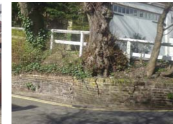
Damaged retaining wall
