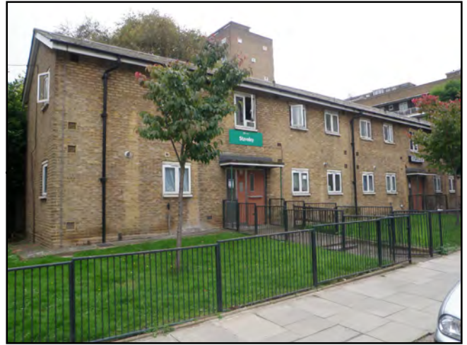
Photograph 6: Suitable roosting features, including a lifted ridge tile, were identified on the Stavely Overbuilds (Building 6), which was also assessed to have low potential to support roosting bats.
