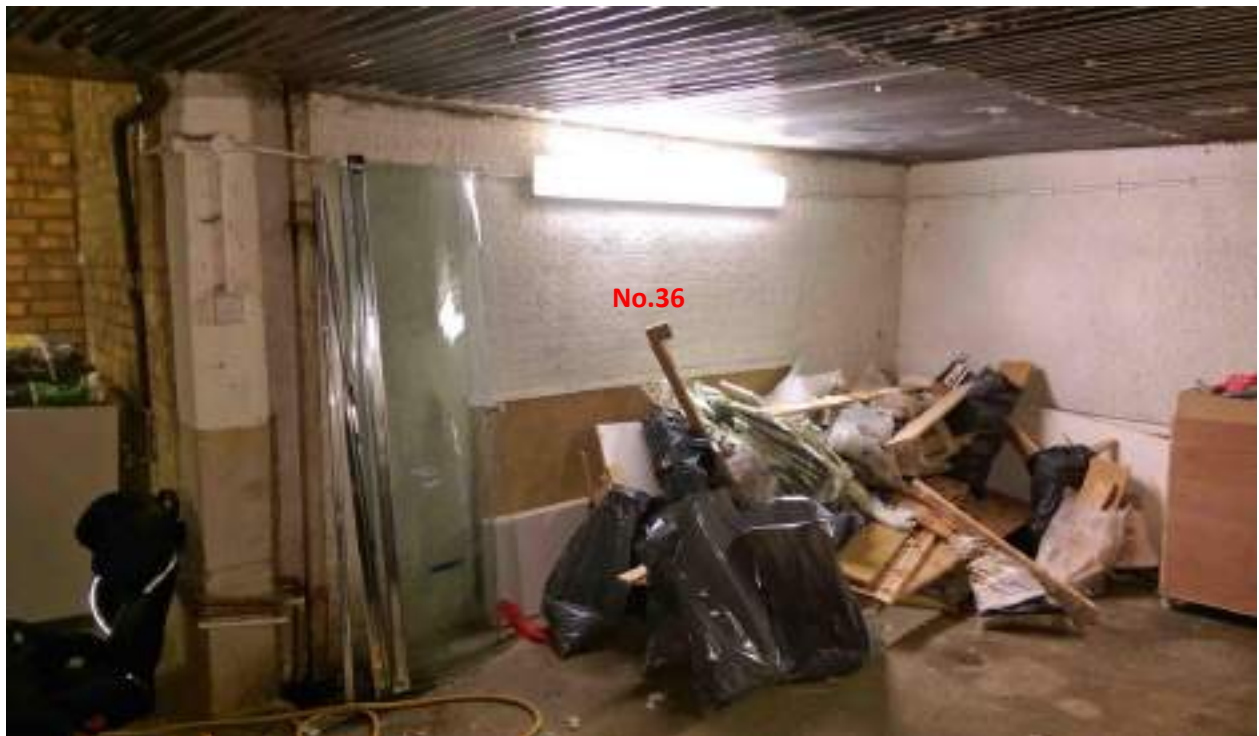
Photo 6: The communal parking area is located behind No.36, underneath the patio area (photo 5). The depth of the proposed basement will exceed that of the parking area, therefore the rear wall of No.36 will need to be underpinned. Note concrete pillar on left.
