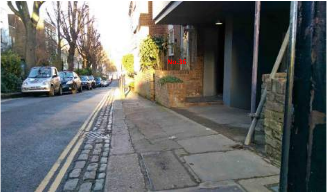
Photo 3: The footway falls gently towards the carriageway in front of the property, and falls more steeply towards the carriageway at the cross-over to the communal parking area.
