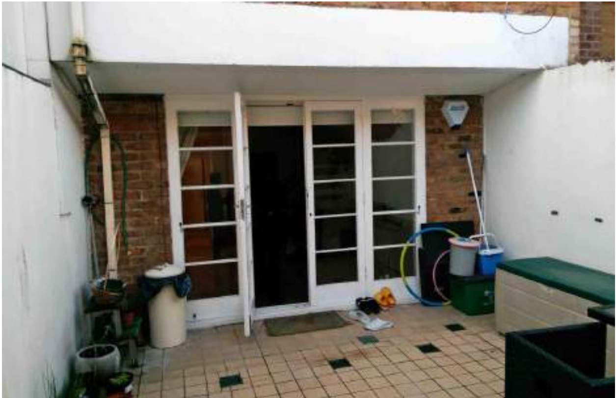
Photo 7: To the rear of the property a concrete beam can be found spanning the width of the house, resting on the No.36/34 and No.36/38 party walls. This beam transfers the load of the rear wall onto the party walls.
