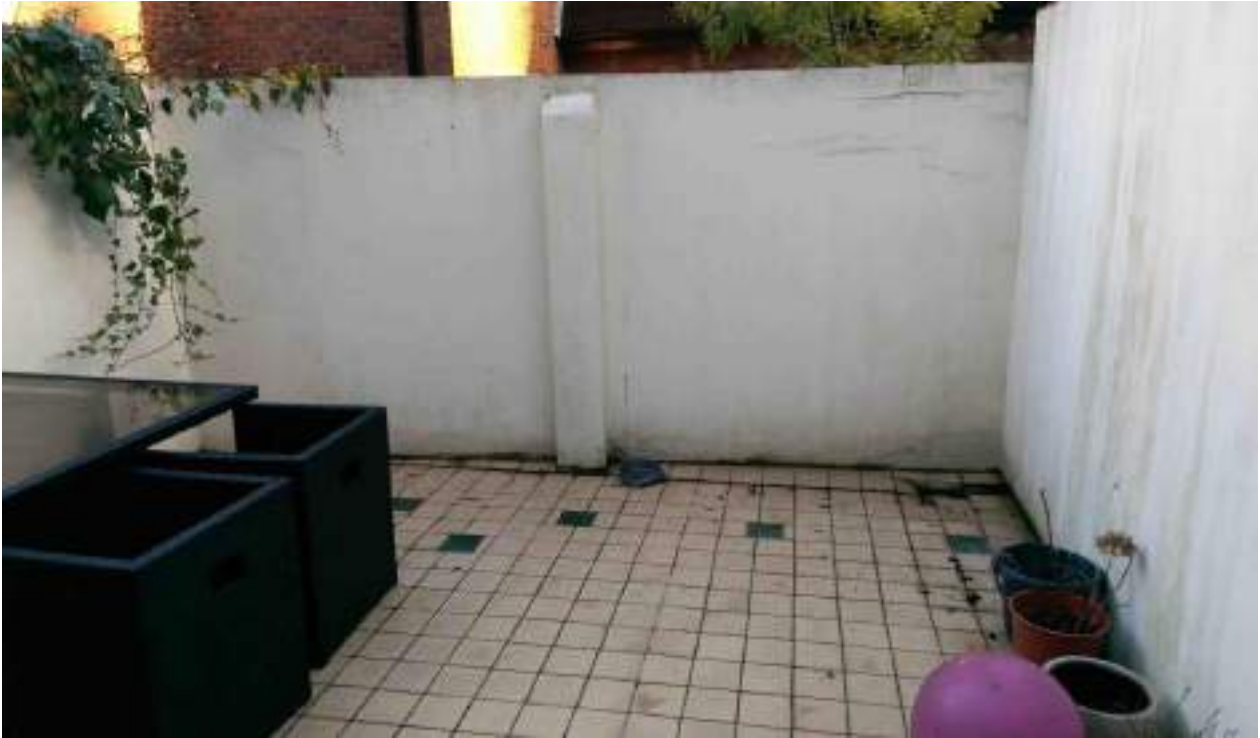
Photo 5: To the rear of the property there is a courtyard patio area which is bounded by high rendered walls on all sides, and surfaced with tiles.
