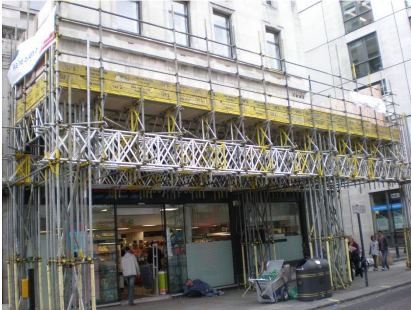
Typical Loading Gantry
