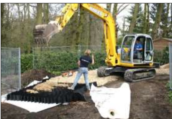
Photo 11: Cellular products are a very effective means of providing ground protection where heavy vehicle use is expected. Here, it is being used to temporarily widen an existing road, to be removed once the construction is finished.
