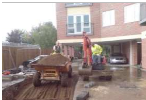
Photo 53: Structural tree soil retains sufficient structure for tree roots to grow, even when compacted.
