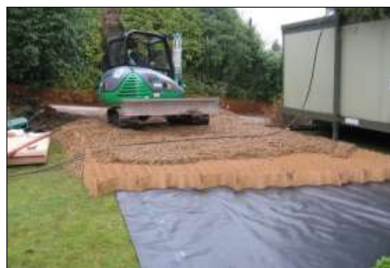
Photo 25: The stone-filled cells spread the load of traffic and the geotextile membrane on the ground prevents migration of the stone into the soil profile.
