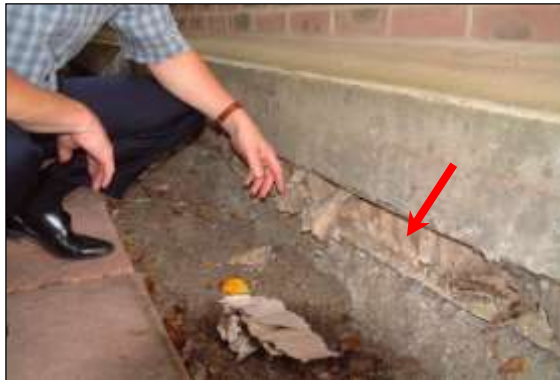
Photo 42: Where a slab is cast on site, a biodegradable void-former (red arrow) temporarily supports the weight of the liquid concrete until it sets. The void-former can then be wetted and washed away to leave a void or left to degrade naturally, both of which allow movement of air beneath the slab.
