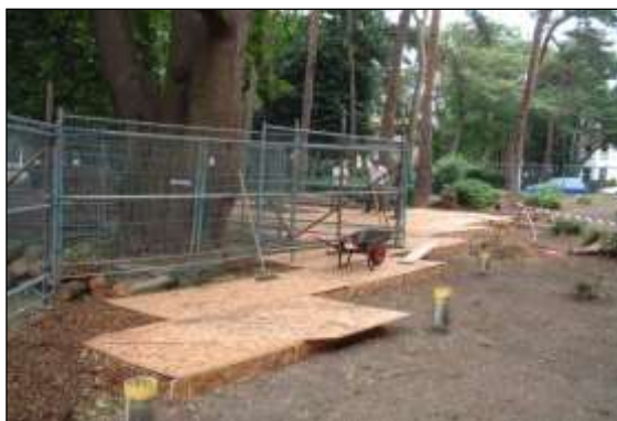
Photo 40: Once the piles have been installed (yellow tops), the ground protection to support the piling rig is removed ready to fix the void-former onto the bare soil, in advance of pouring the building slab.
