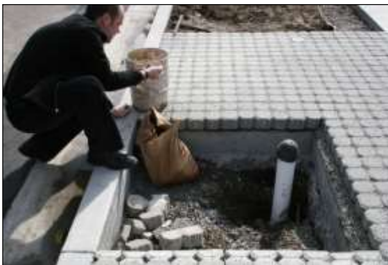
Photo 57: The finished surfacing is profiled to leave the tree pit open, ready to be filled with good quality topsoil and the new tree.
