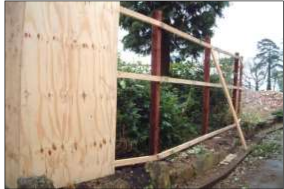
Photo 4: Board specification on secure wooden posts is a suitable alternative to the standard braced scaffold design.
