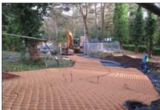
Photo 24: The three-dimensional cells are opened up, spread across the area to be surfaced and pinned in place ready for the stone filling.
