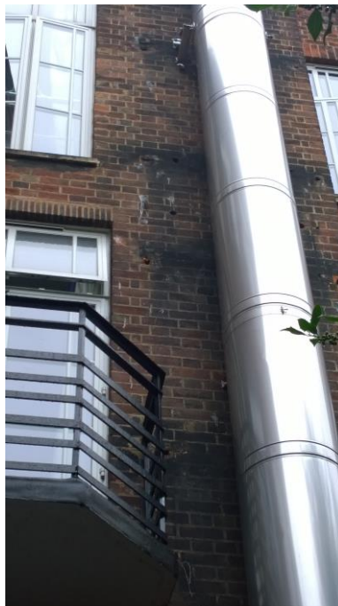
Photograph 10 Gaps in masonry created by removal of external fixtures on eastern elevation of B1.
