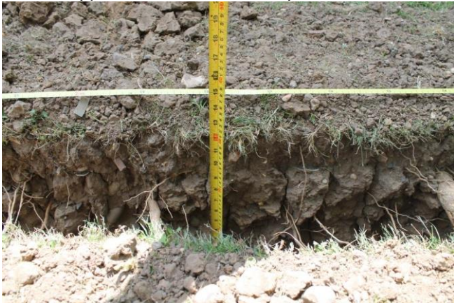
Photo 8. Ground was very hard clay. Even after terraventing to break up the soil the excavation had to cease at approx. 300mm -350mm depth
