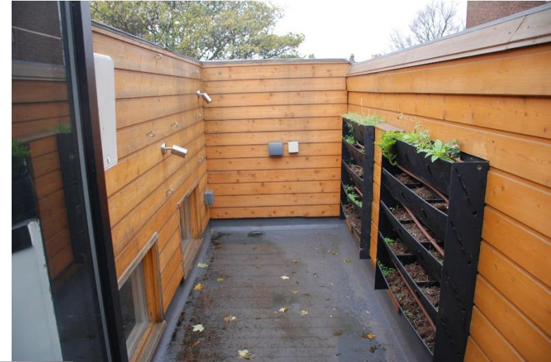
GRP roof terrace within existing roof space, to be removed and covered over for mansard.
