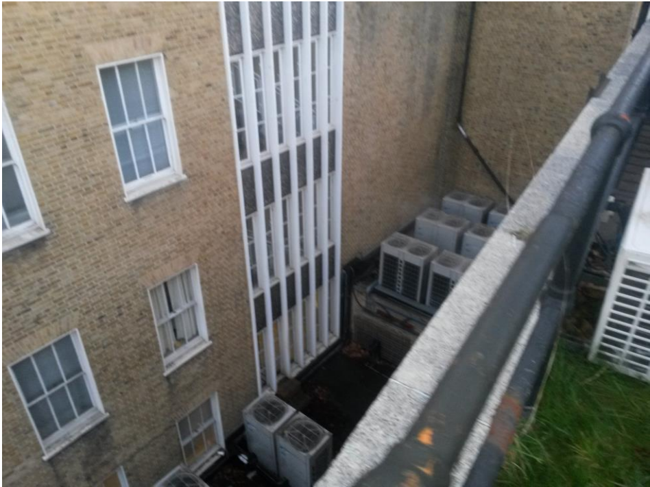
Figure 7 – External plant at the rear of 175-185 Gray's Inn Road
