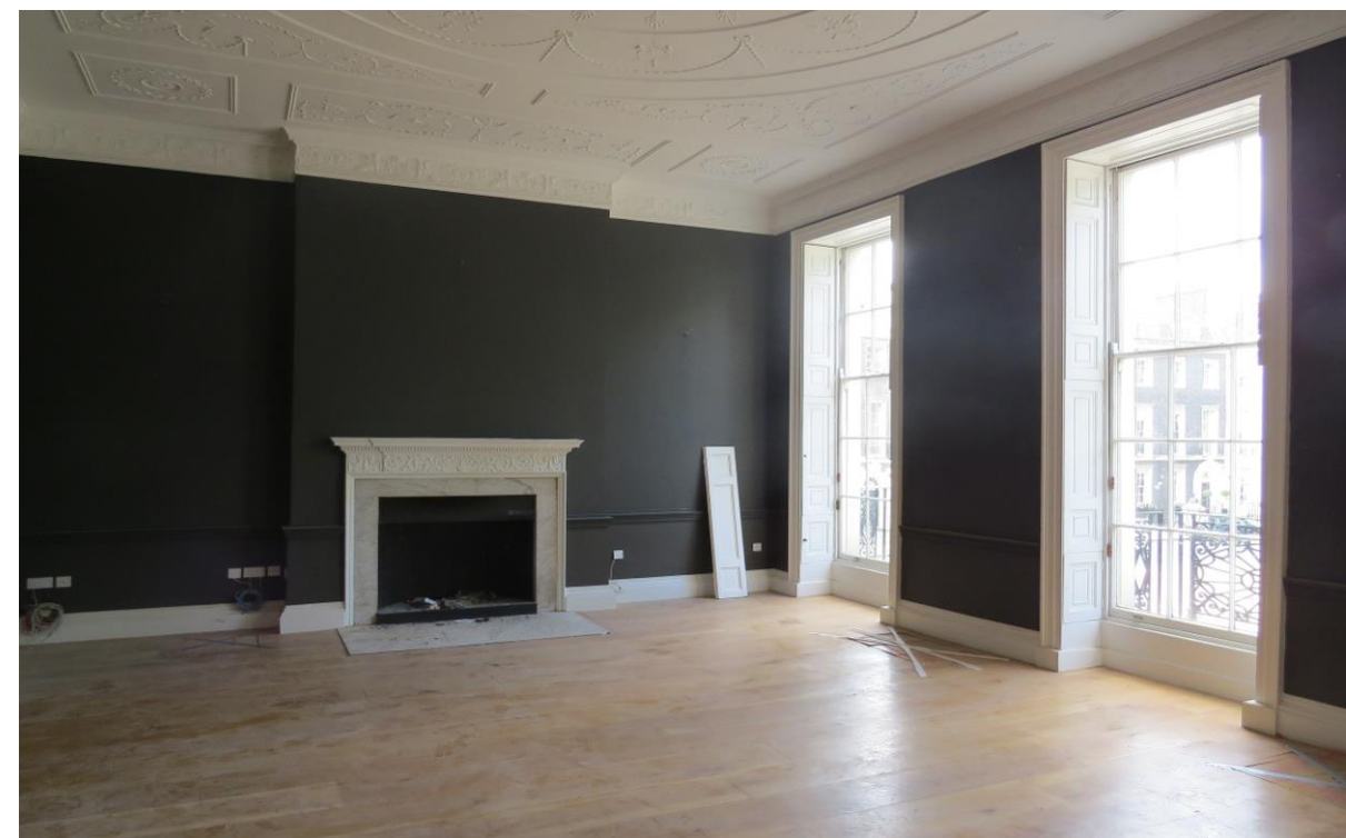
Fig. 7. The First Floor front room showing the floor to ceiling sash windows.
