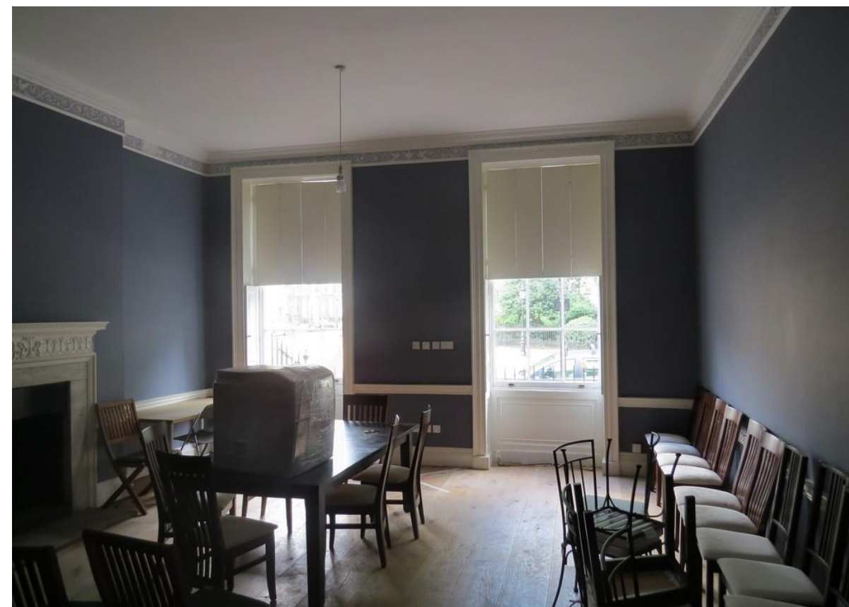
Fig. 6. The windows in the front room at the ground floor level, showing the original shutters.
