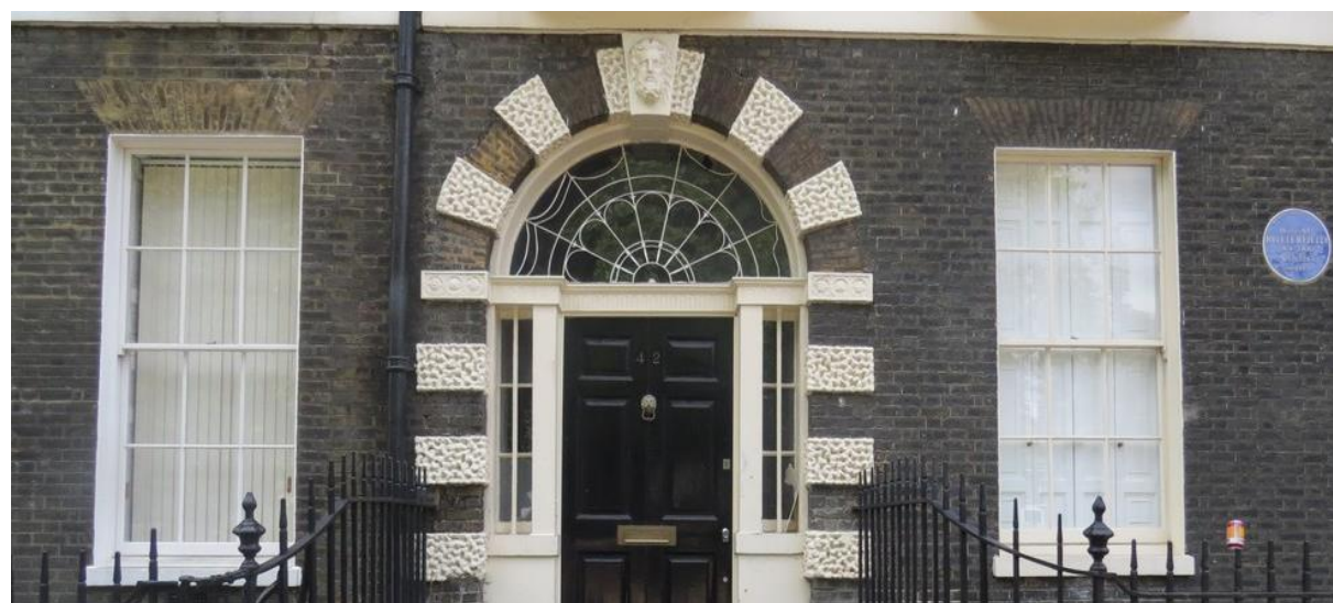
Fig. 5. The existing ground floor recessed timber sash windows, and the arch headed fanlight above the entrance doorway as seen from Bedford Square.
