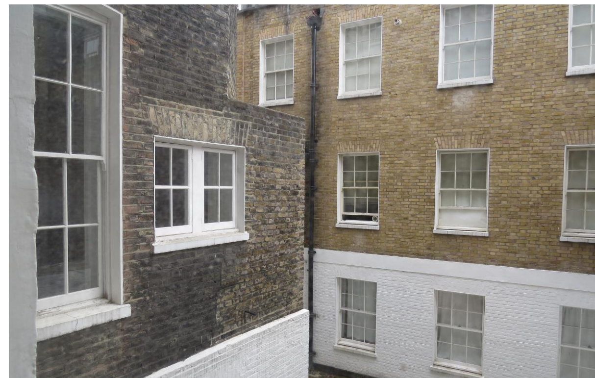
Fig. 12. Courtyard to the rear of the main house, showing the base of the closet wing and the rear elevation of the mews.
