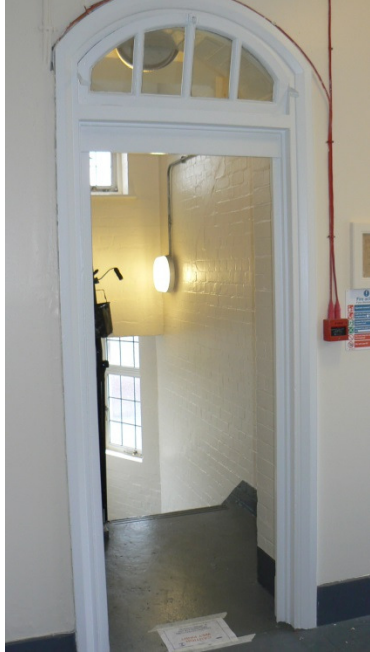
4 th floor landing door frame. New door to be fitted within existing frame.
