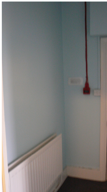
LFB offices' side of the wall where opening is to be formed.
