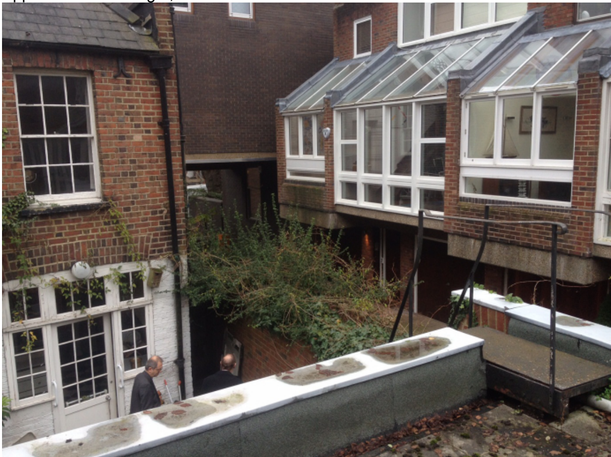
View back to main house with Lakis Close properties to the right
