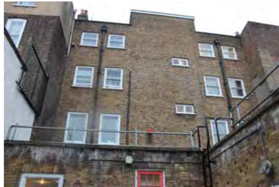
FIG 27. REAR ELEVATIONS TO NOS.14 AND 15
