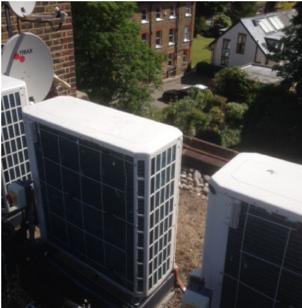
Photo 5: Central flat roof area – air conditioning units and satellite dishes (brown roof behind)
