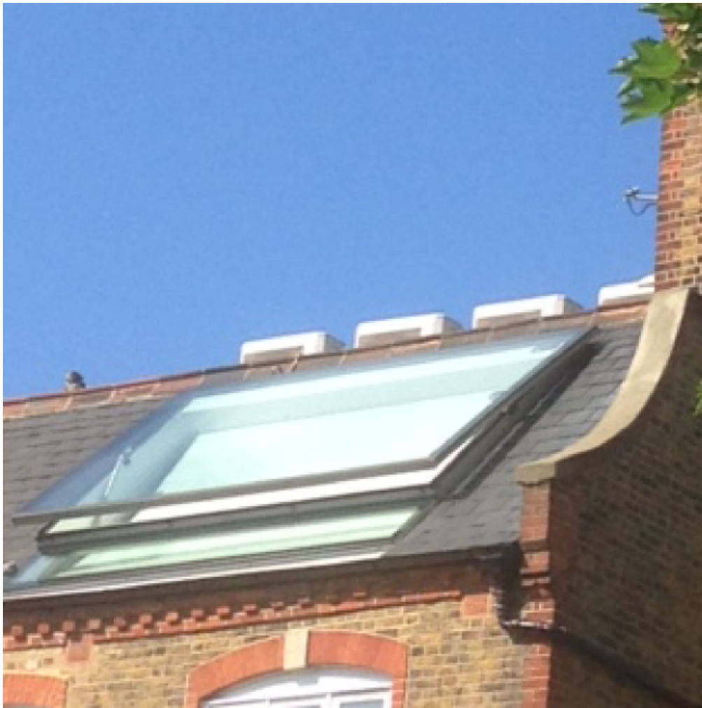
Photo 4: Rear of property #2 – view from neighbouring car park (rear sloping part of roof)
