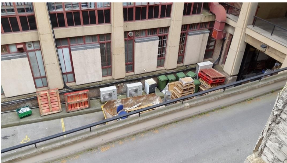
Figure 7: Other condenser units in the loading bay, viewed from the logger position
