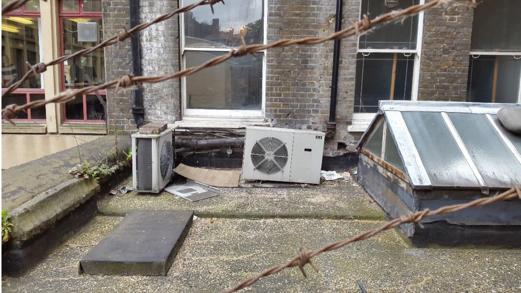
Figure 4: Condenser units close to the noise logger position and directly adjacent to the nearest residential window
