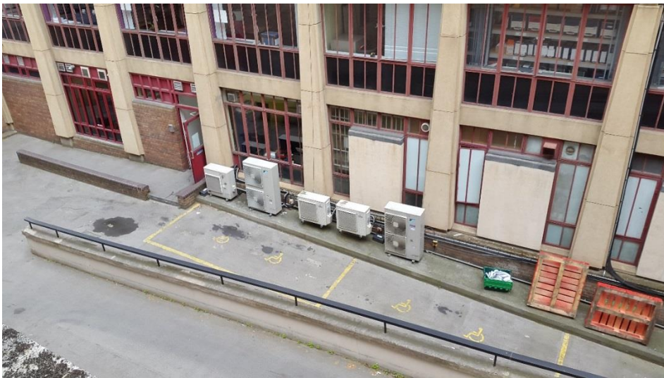
Figure 6: Other condenser units in the loading bay, viewed from the logger position
