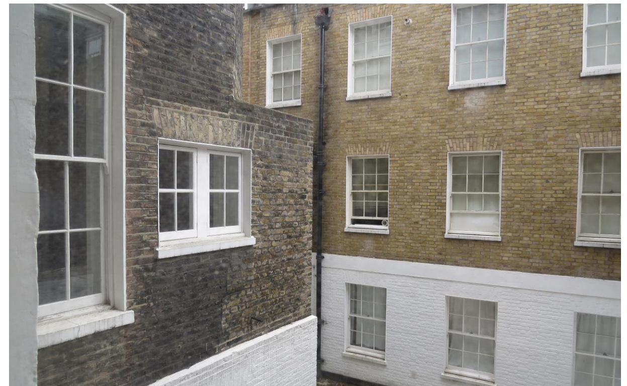
Fig. 12. Courtyard to the rear of the main house, showing the base of the closet wing and the rear elevation of the mews.
