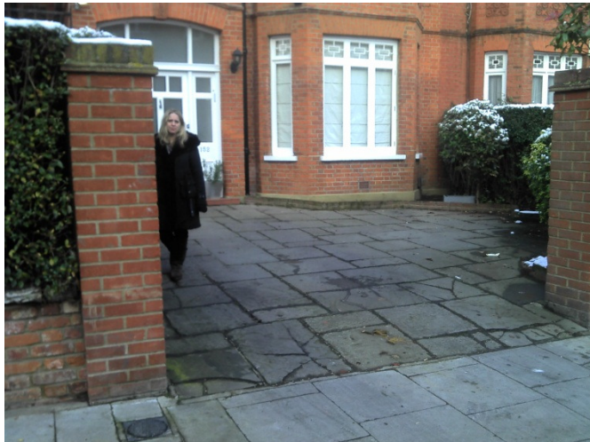
Photo 1: The front driveway design and materials do not enhance the Conservation Area. Some of the paving is damaged.
