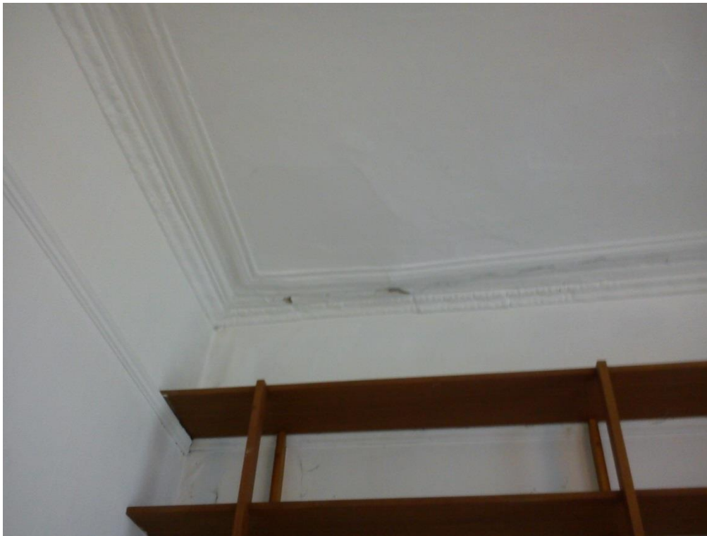
Cornice in rear room that has been damaged, to be repaired
