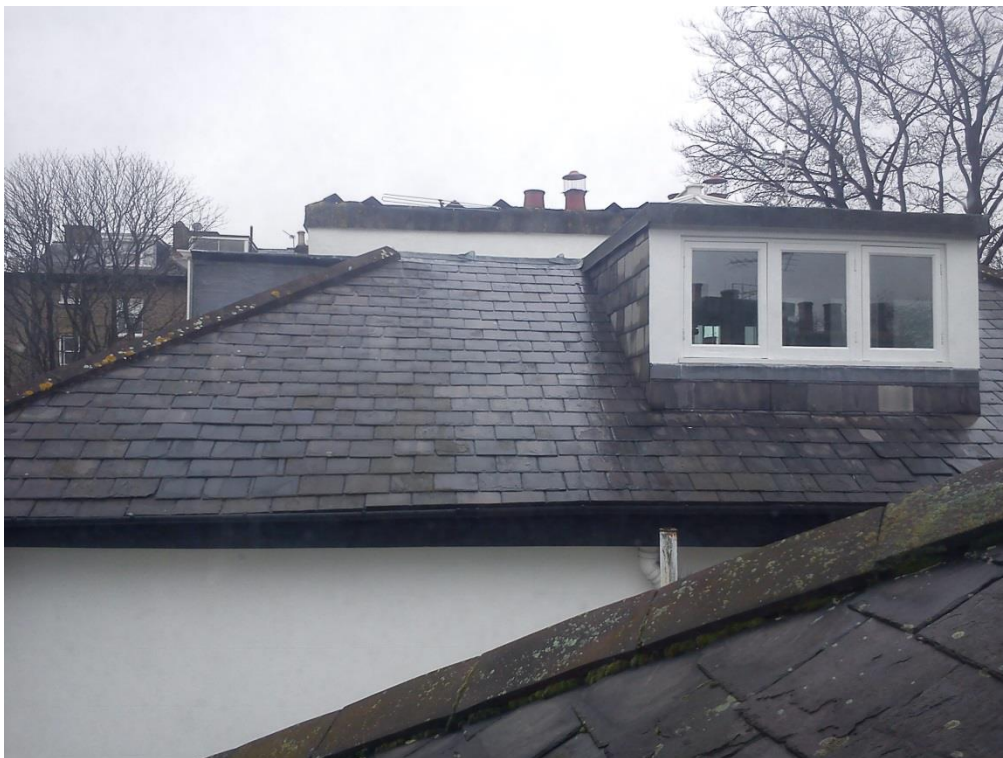
View from roof towards side dormer at No. 17, which it is proposed to broadly replicate
