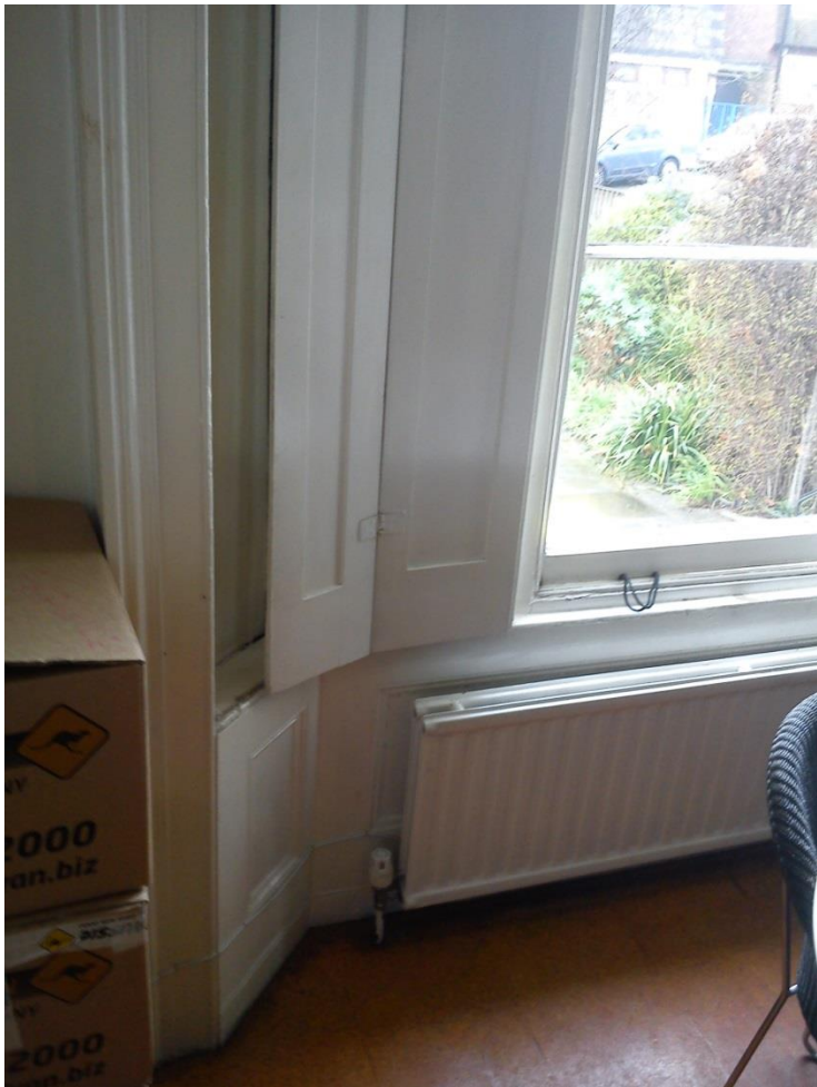
Front room at upper ground floor, showing cornice that will be retained and renovated, and shutters to be retained
