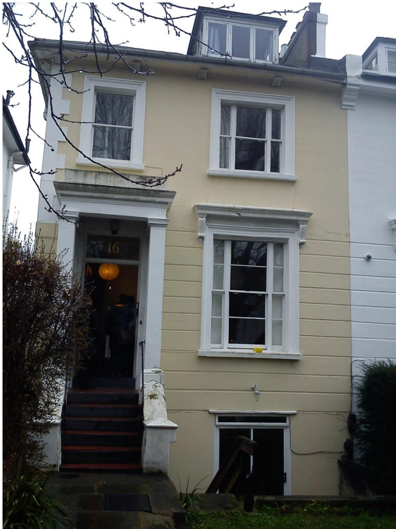
Front elevation of property, showing poor condition to elevation, windows and steps
