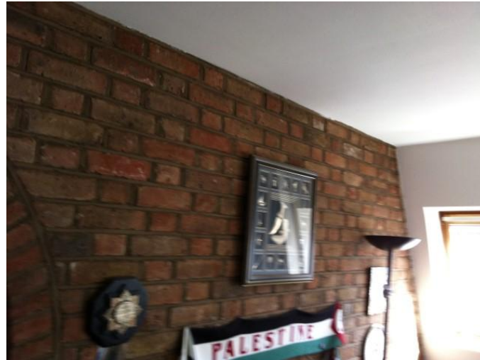
Internal living room wall, to be slightly altered to form stairs to the roof terrace.
