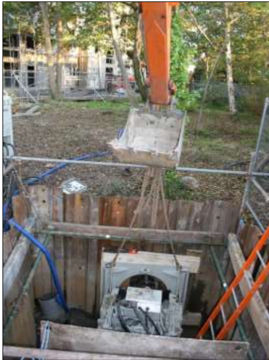
Photo 44: If possible, thrust boring is the preferred option for installing service routes through the RPAs of important trees, but there has to be space at the start and finish to dig substantial working pits.
