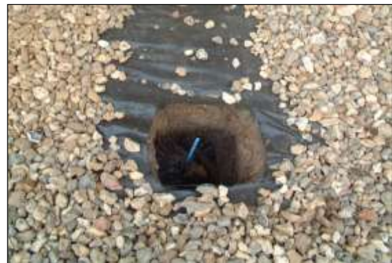
Photo 39: Ground protection must be used to spread the load of the piling rig once excavation has confirmed that no substantial roots are in the preferred pile location.
