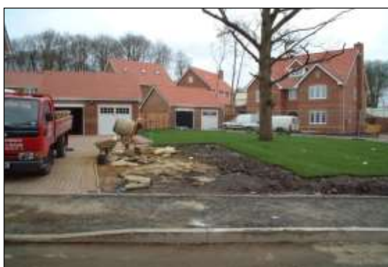
Photo 48: The RPA of this tree was not effectively protected during construction and excessive compaction of the soil meant it died soon after this turf covered up the damage.
