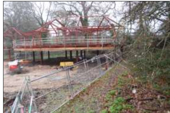
Photo 37: It is possible to support very large structures on piles within sensitive RPAs without any significant adverse impact on tree roots.
