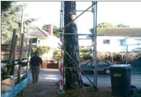
Photo 5: A scaffold braced framework surrounding the trunk reduces the risk of accidental impact.
