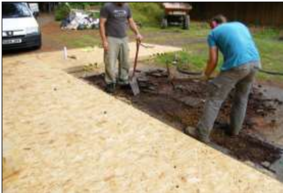
Photo 15: Careful hand-digging using conventional tools is acceptable for exposing roots in RPAs.
