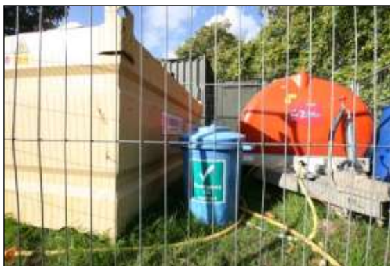
Photo 46: Where fuel or other chemical are stored on site, it is now standard practice to have emergency spillage kits available to restrict the environmental impact of accidents.
