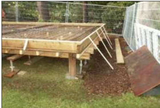
Photo 36: Small diameter piles (less than 150mm) are an effective means of supporting structures in RPAs with minimal disturbance.
