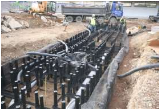
Photo 55: The individual Silva Cells can be assembled in layers and service ducting threaded through before filling with soil and fitting the reinforced tops.
