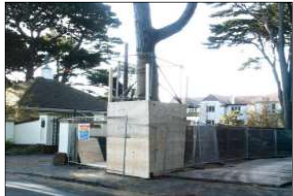
Photo 6: Board secured to scaffold framework adds another layer of protection for vulnerable trunks and branches.
