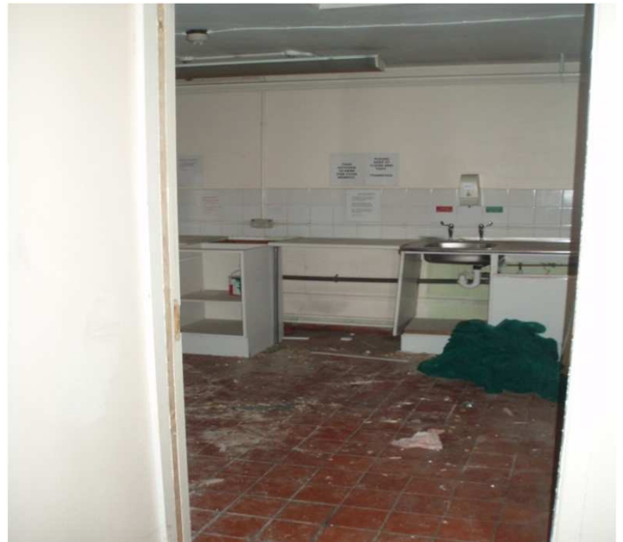
Image 14: Kitchen in poor state of repair (Disused Building)
