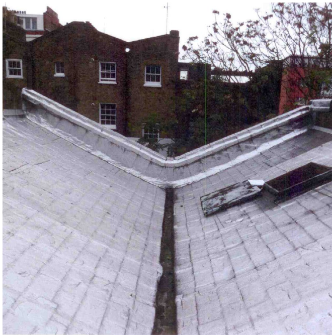
fig20. Roof with 'flashband' covering
