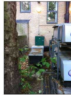
Photograph 2 Existing WC Extract Fan
