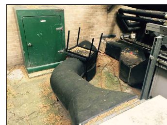
Photograph 5 Existing Low Level Extract Ductwork
