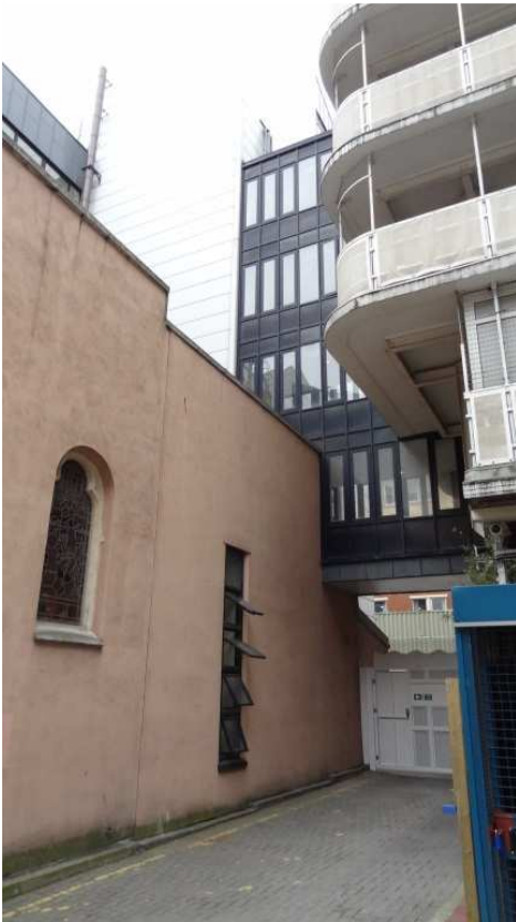
Figure 7: View of the chapel from the hospital courtyard, showing the joint line between new and construction
