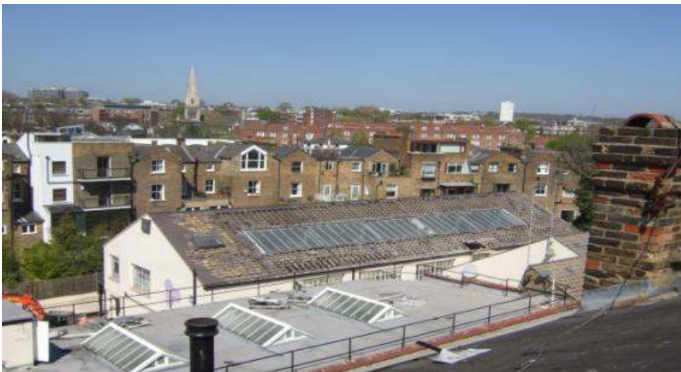
Above: View from the rear roof slope of 99 Regents Park Road showing the variation of roof extensions
