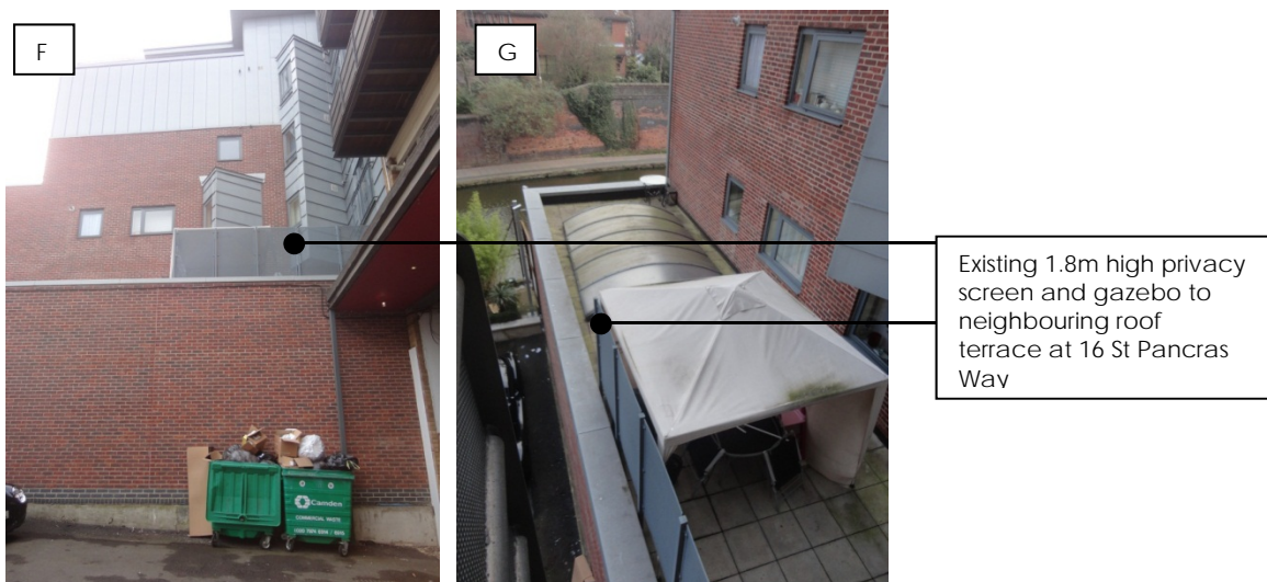
Image F: View from rear courtyard looking up to No.16 roof terrace at 1.8m privacy screen. Image G: Looking down onto No.16 roof terrace (Photos taken March 2015)
