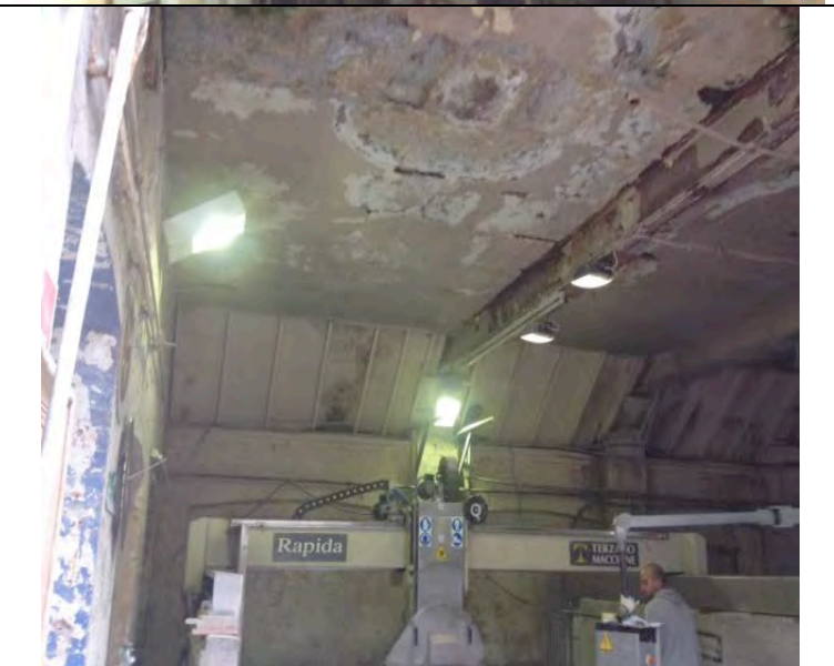
Photograph 3: The inside of one of the buildings with machinery present. Note the apex of the roof exposed.
