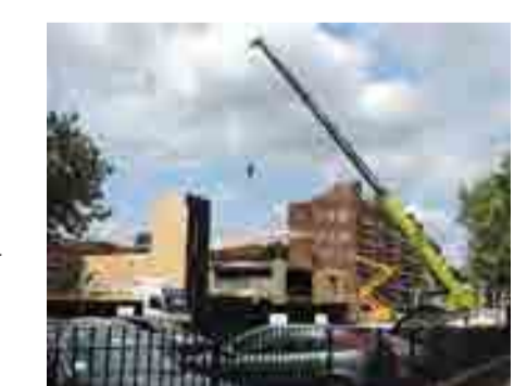
Frampton Park Baptist Church A new baptist church in Hackney constructed from Cross Laminated Timber. The structural elements are pre-fabricated off site and craned into place, allowing the building to take shape quickly. The construction method is very air tight and thermally efficient, making it very sustainable.
