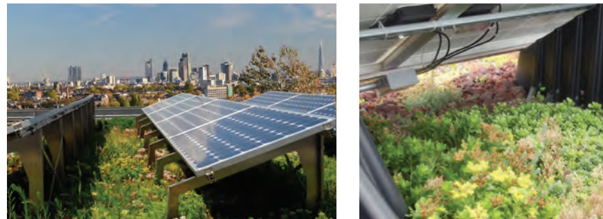
PV panels provide shading which supports micro-habitats on extensive biodiverse roofs
