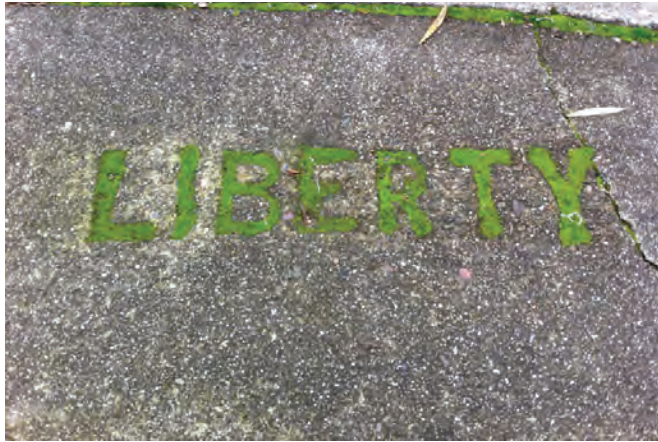
Moss text in in-situ concrete slabs
