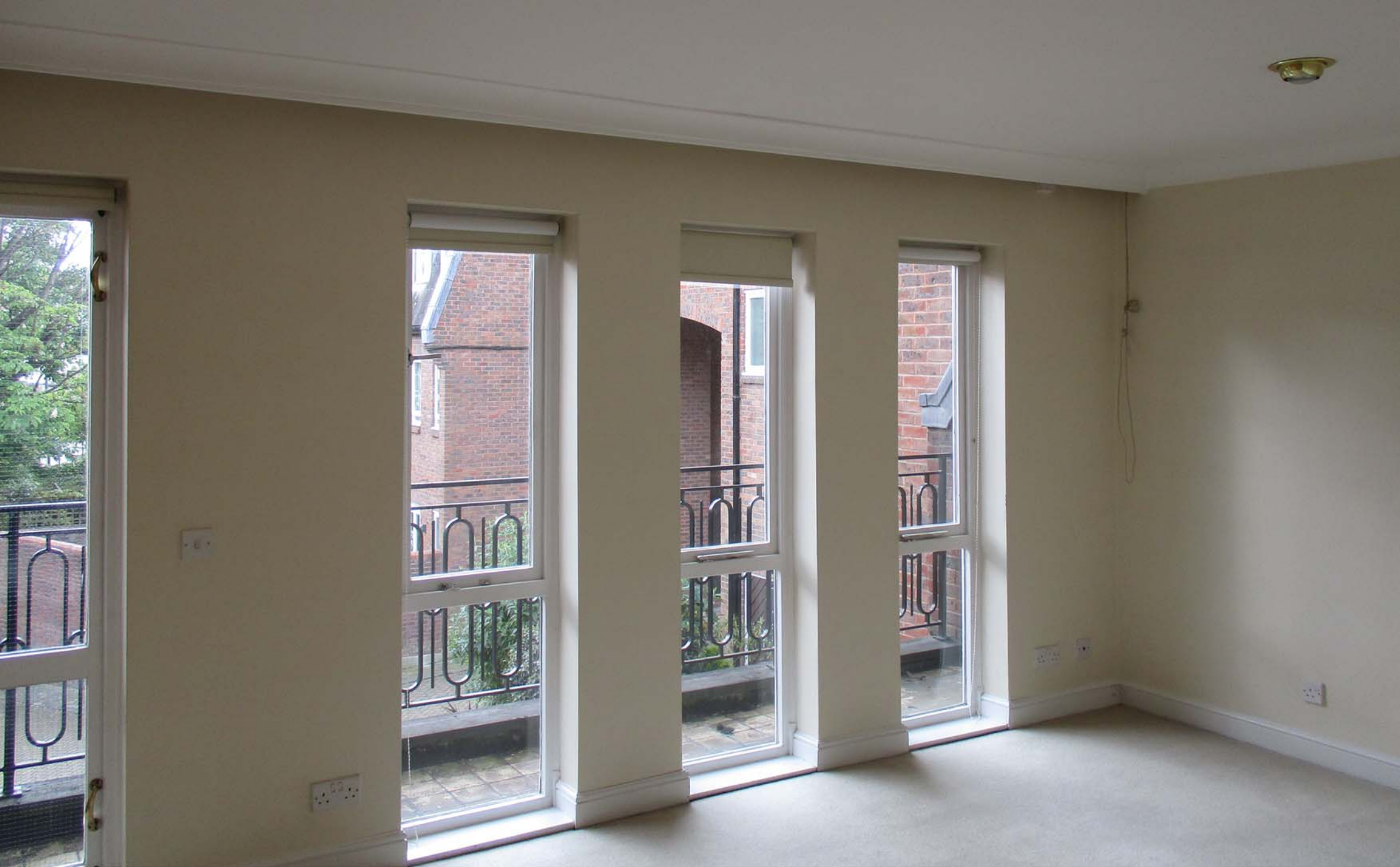
site photos : master bedroom : first floor front : note georgian wired glass side hung window + double glazed side hung windows with fixed lower pane
