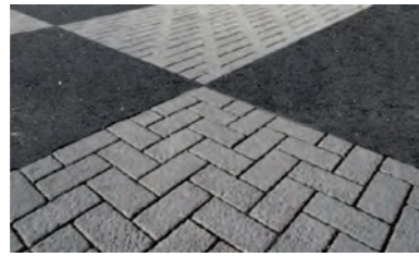
2. Large chequerboard of asphalt and silver grey high quality setts to meet LBC adoptable standards
