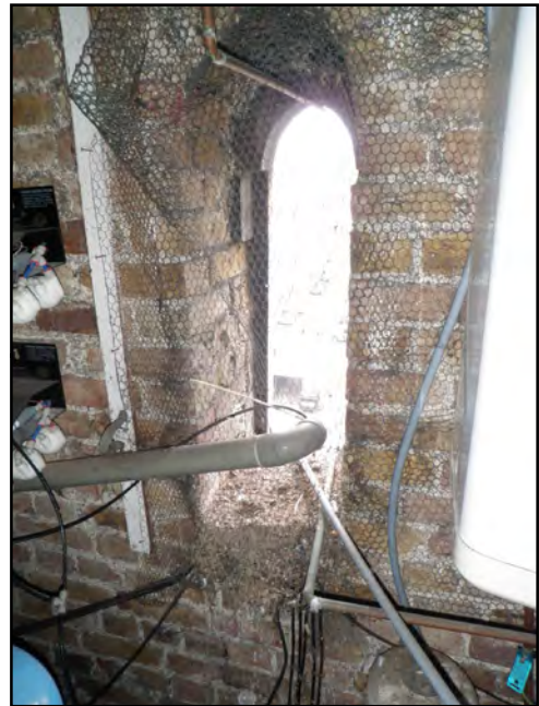
Photograph 4: St. Bede's Hall evidence of breeding birds within the elevated tower section to the south.
