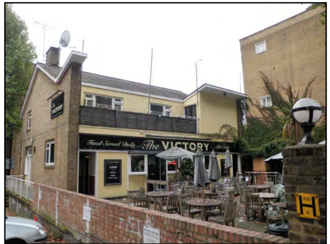
Photograph 8: Missing and loose roof tiles were recorded on the roof of the Victory Pub (Building 8) which was assessed as having low potential to support roosting bats.
