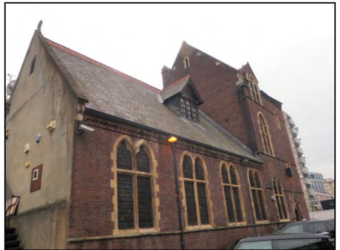
Photograph 4: St Bede's Hall (Building 4) is a former church, structure assessed as having low overall potential to support roosting bats.
