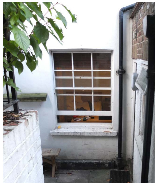
Existing lower ground floor window to be removed, opening enlarged to floor level.
