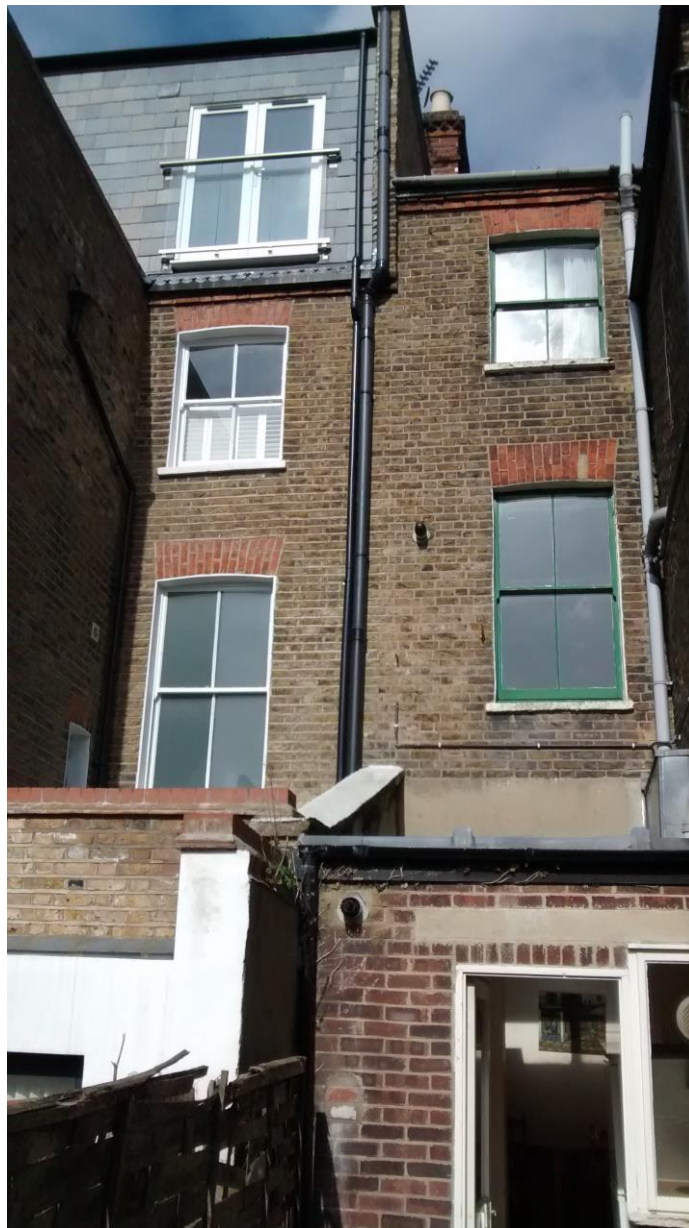
Figure 1 – Rear picture of the above-addressed property and number 21 on the left side
