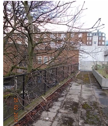
Photo 7: Overhanging canopy of T6
