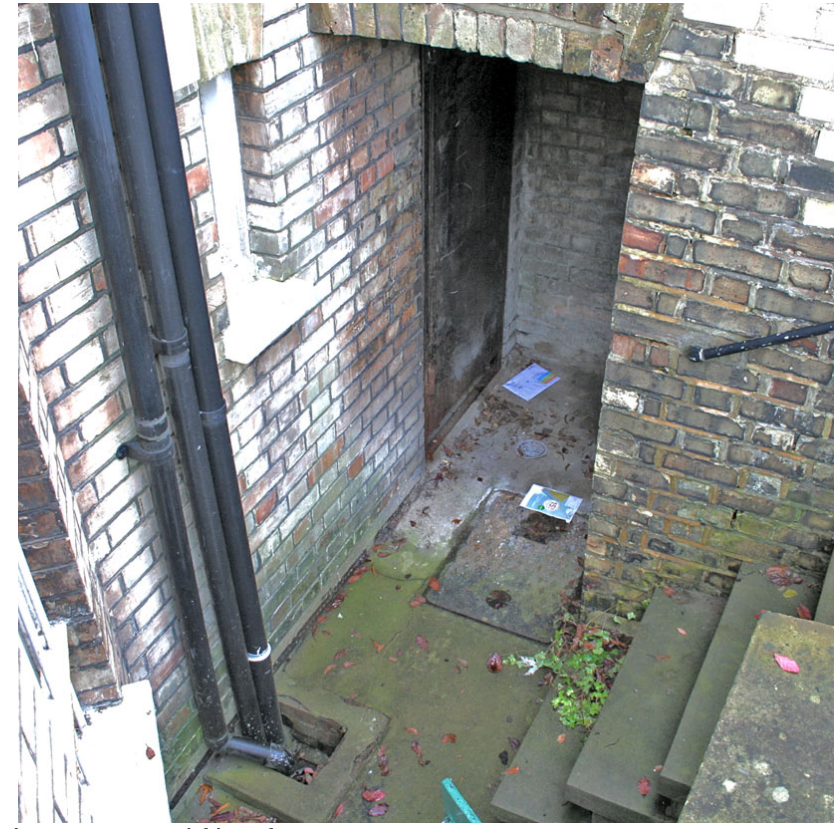
Lower ground floor front access to No.2 Gayton Crescent and to Vault 1.
