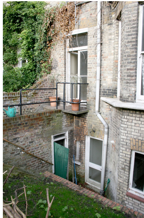
Access to Rear Garden from Ground and Lower Ground Floors at No.2 Gayton Crescent.
