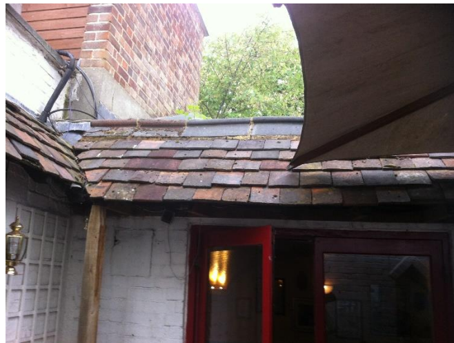
Canopy to be removed in courtyard
